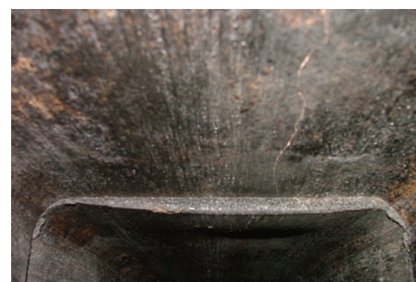
A crack like this can allow deadly gases to leak into the home, and can open the way for a chimney fire to turn into a house fire
