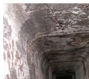
Cracked flue tile
