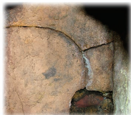
Damaged flue: Notice the moisture and the missing piece of flue tile.
