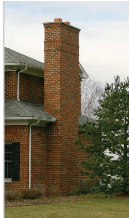
This chimney may look fine on the outside, but what about the inside?
